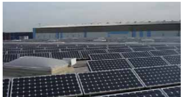
Neska's new solar facility promotes renewable energy.
