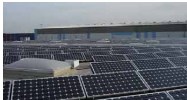
Neska's new solar facility promotes renewable energy.
